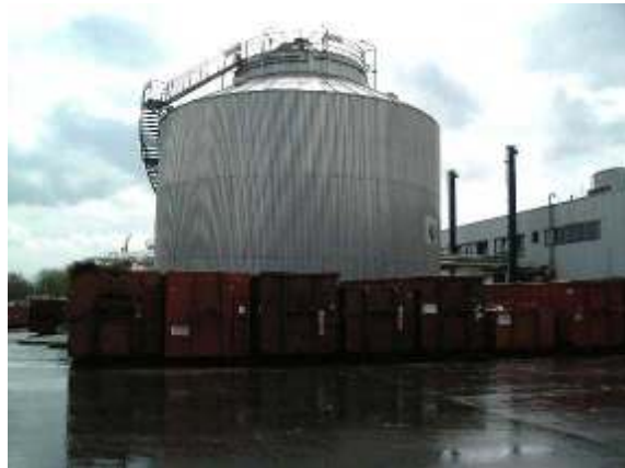
Figure 10 - 3,500m 3 Anaerobic Digester
