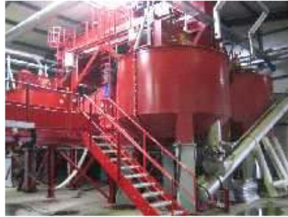
Figure 3 - Waste Dissolver Installation
