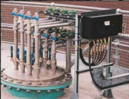
Monsal Biogas Digester Mixing System
