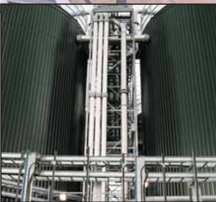
Monsal Biogas Mixing and Transfer system
