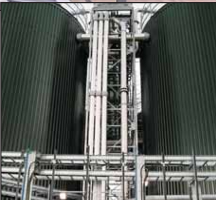
Monsal Biogas Mixing and Transfer system
